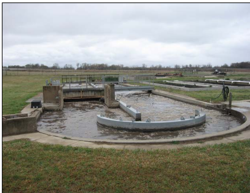
Figure 4.3: Aeration basin and sludge drying beds at the Newark WWTP
