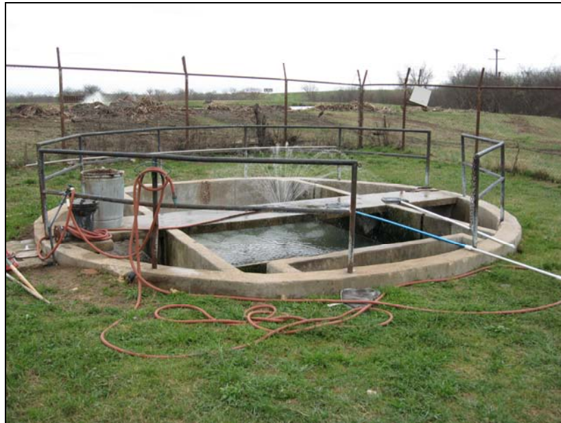
Figure 4.6: An Open-Top Imhoff Tank at the Rhome East WWTP
