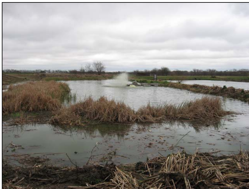
Figure 4.4: Lagoons at the Rhome East WWTP
